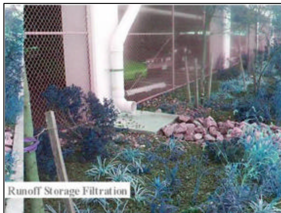
Downspout disconnection into vegetated area Source: LID Center
