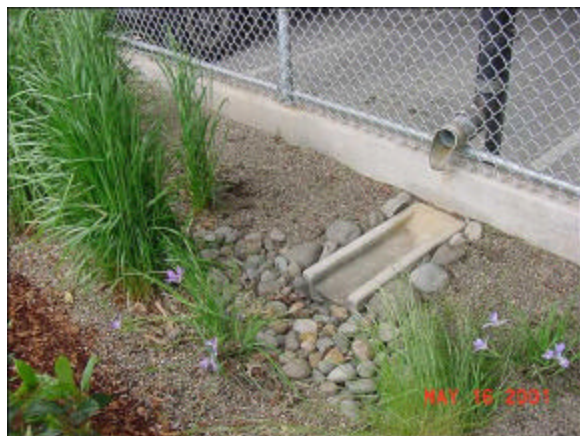
Downspout disconnection into vegetated area Source: PGDER
