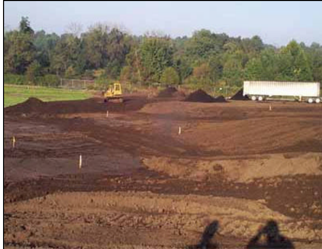
Southern Maryland Wood Treating Site: Final Grading and LeafGro Placement Source: U.S. EPA
